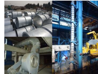
Ductwork Steam Exhauster up to roof
