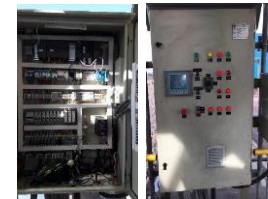
LOCAL CONTROL PANEL
