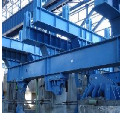
Turn over Cooling Bed
