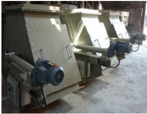
Motorized Diverter Gate
